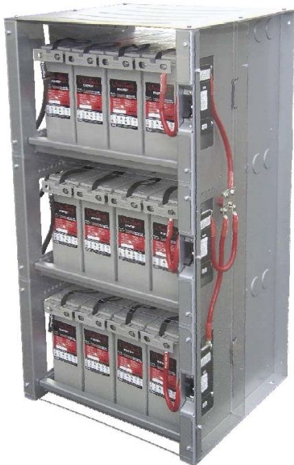
25kwh Battery Bank
